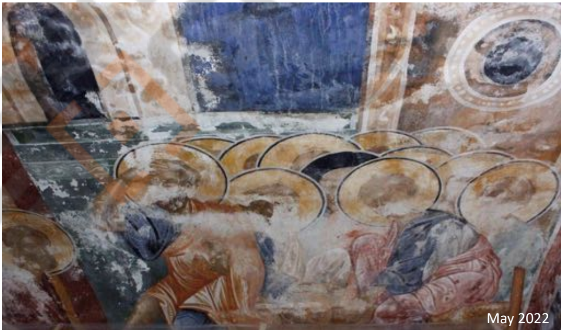
Figure 3a, 3b and 3c. Images of the west arm vault, south side in December 2017, March 2021 and May 2022 show the severity and ongoing nature of the current deterioration due to moisture and salt activity.
